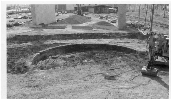
Portion of retaining wall for turntable pit, New Haven rail yard roundhouse, 1870. Piers in background are for the Church St. overpass.
